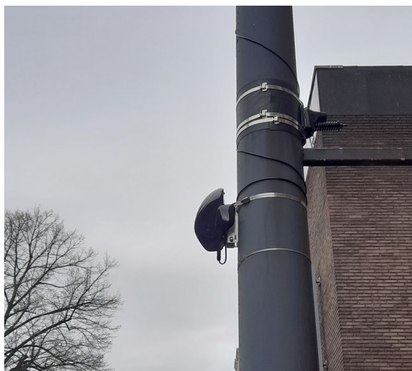
Figure 1 - Vortex Automatic Sensors
